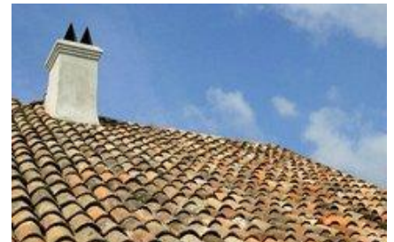
STAFF PHOTO BY CHRIS GRANGER The Colombian barrel tiles crown a Creole cottage on St. Ann Street in the French Quarter.
