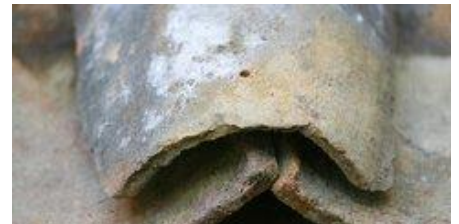
STAFF PHOTO BY CHRIS GRANGER The Colombian barrel tiles are laid in an overlapping, over-under pattern and are secured with copper wire.
